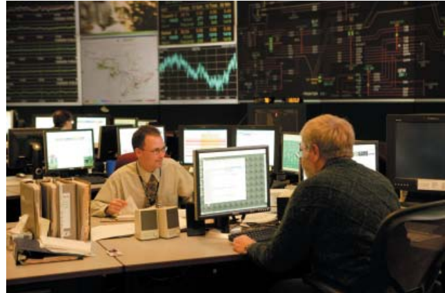
IESO Control Centre
